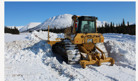
Dozer on standby for snow clearing at a staging area for the clearing and drill crew off West Juneau Creek Access Road.
